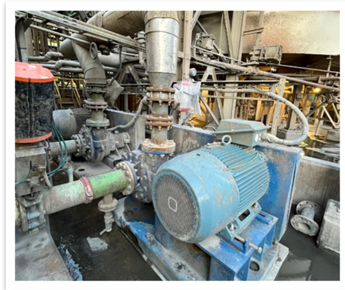
Figure 1- Process Water Pump
